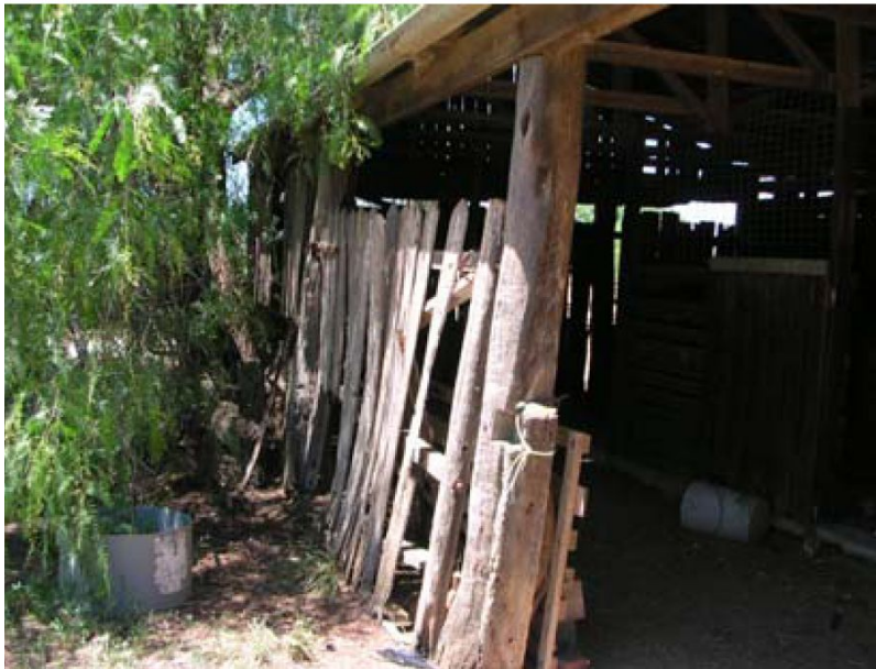
Stable building 1- This structure has been constructed using a variety of building techniques and materials. The structure is eclectic and cobbled together in a relatively ad hoc manner.
